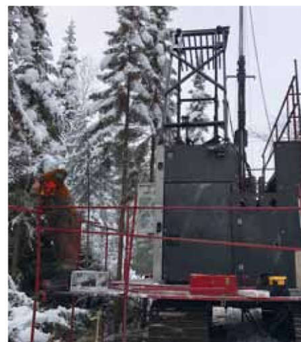
Sayona continues to work closely with the Quebec Government, which is firmly focused on developing its own battery supply chain
